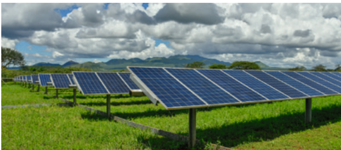
Solar panels installed at the Kilaguni Serena Safari Lodge, Kenya. © GIZ/James Ochweri
