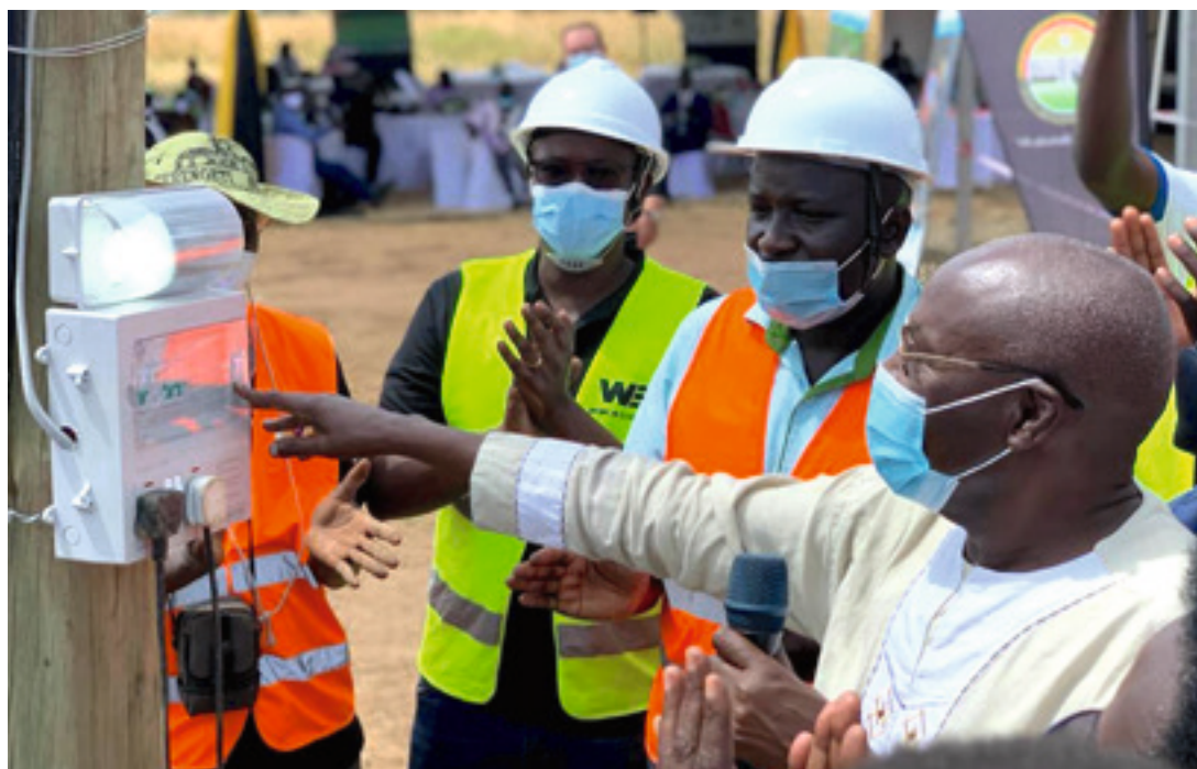
Commissioning of solar mini grids in Northern Uganda. © GIZ Uganda/Energy and Climate Cluster
