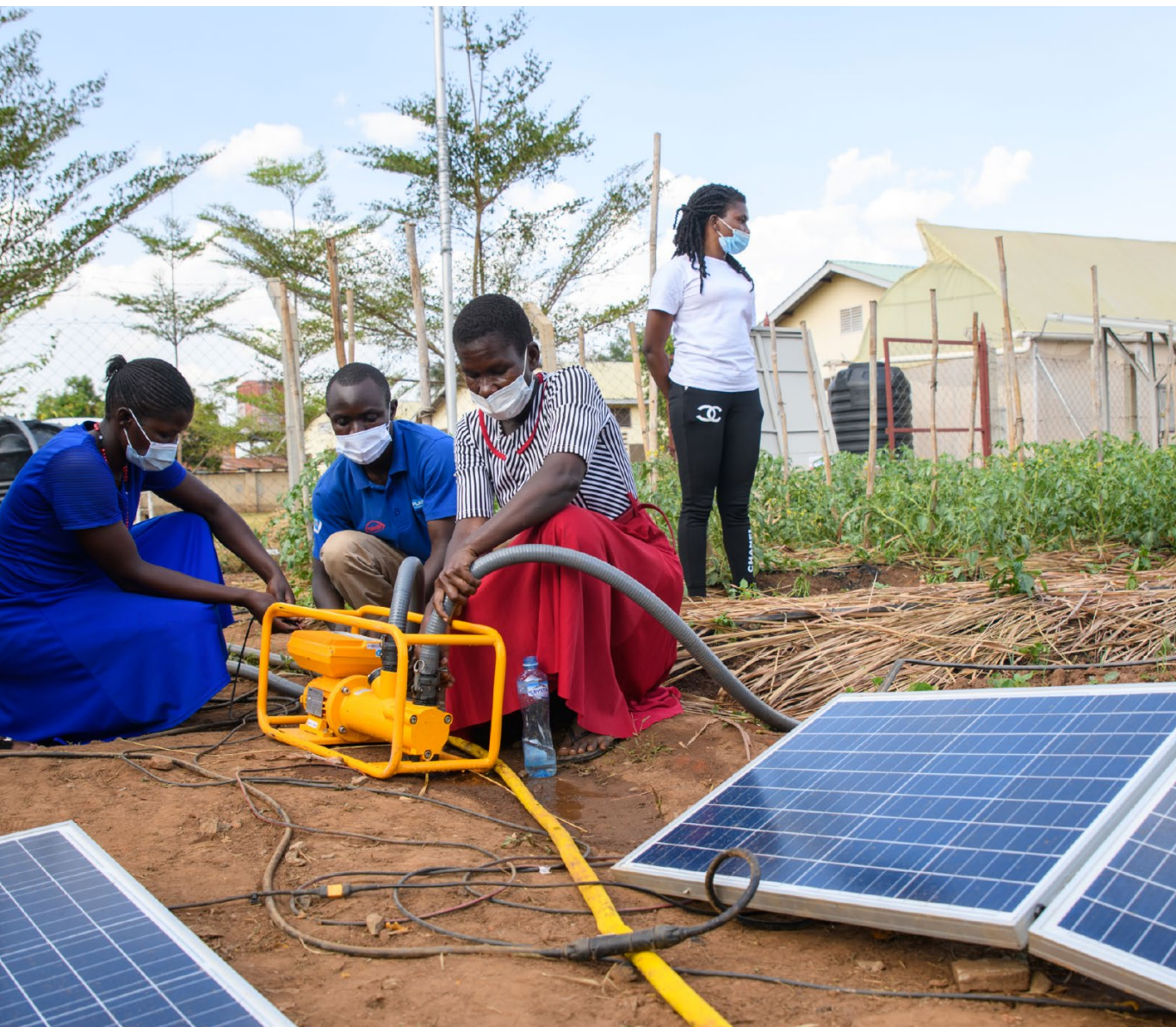
Training for solar powered irrigation systems in Uganda, GIZ project Green People's Energy for Africa. © GIZ
